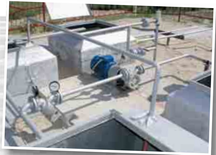
Underground autogas installation using one autogas series pump with two tanks.
